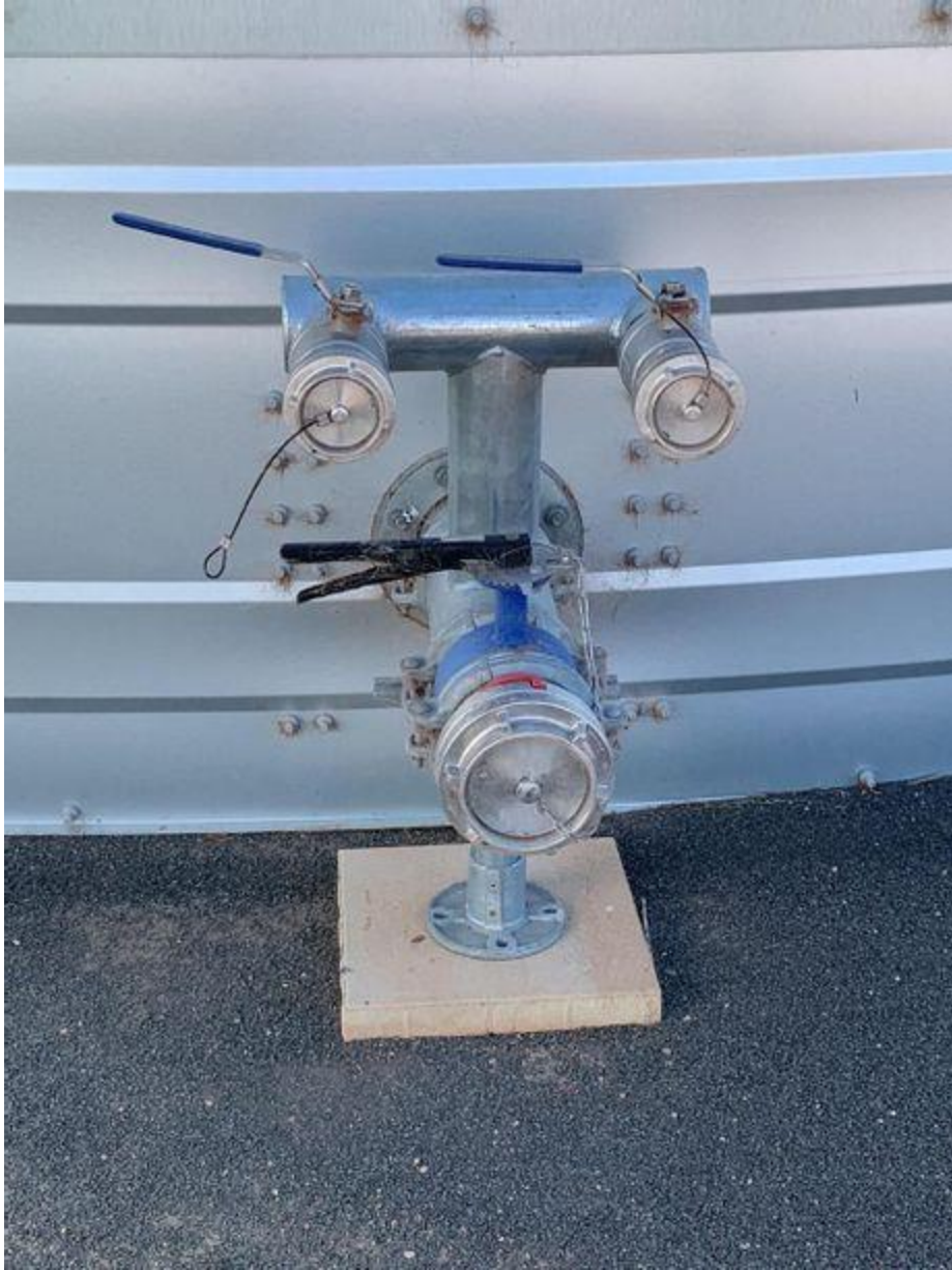
Farm 79 - Connection on water tanks for RFS to connect to for fire response
