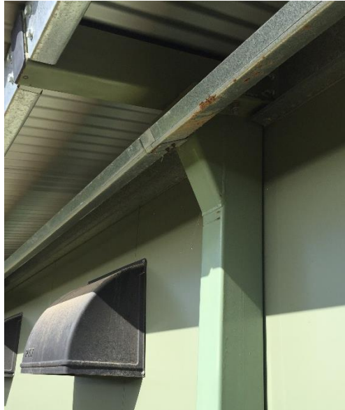
Figure 4: Example of steel columns on the external face of the EPS panels
