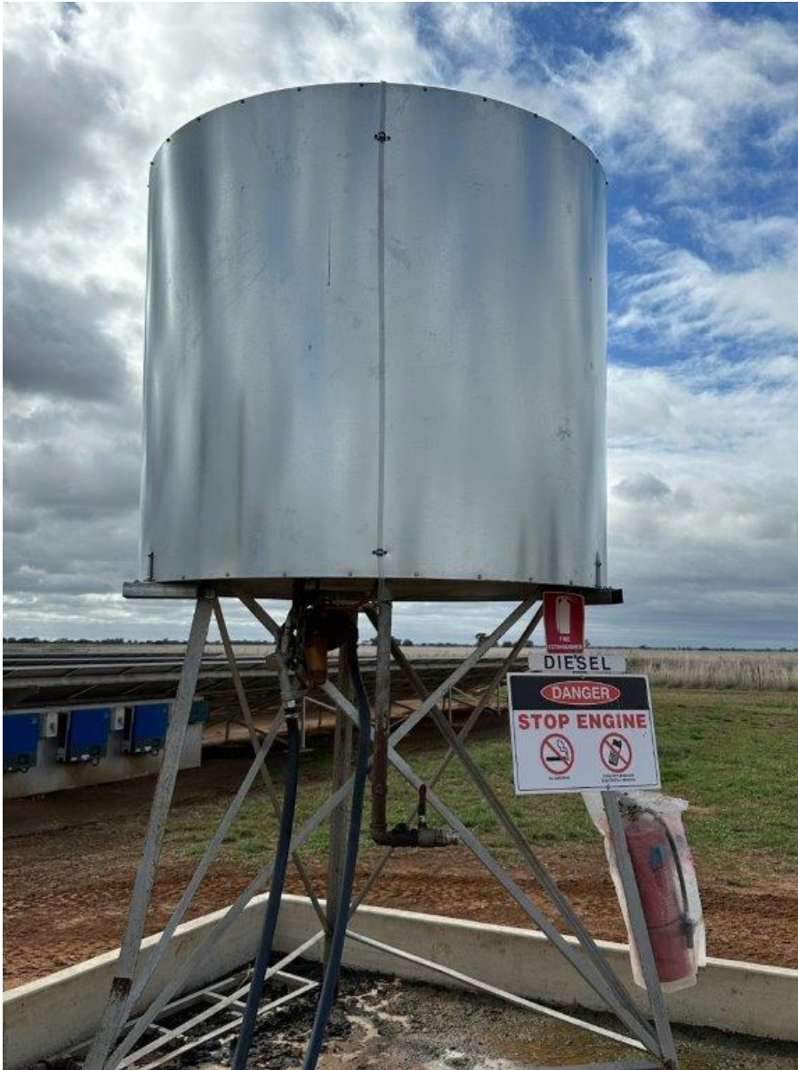
Figure 4 Diesel Tank Shielding
