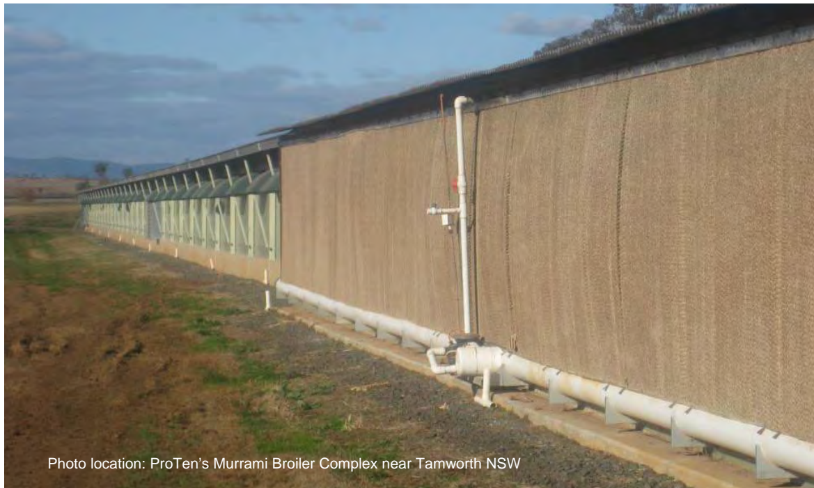
Plate 6 – Broiler Shed Cooling Pad
