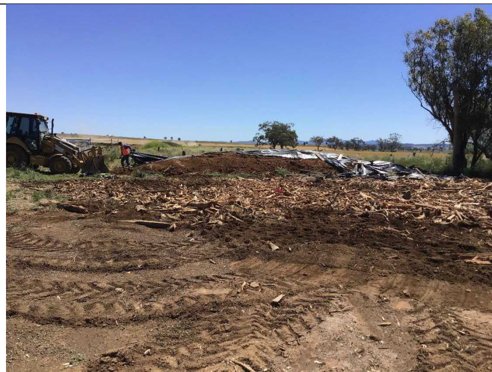
Photograph 21 – Timber stockpile spread and compacted into surface within the remediation area, from adjacent TP 103
