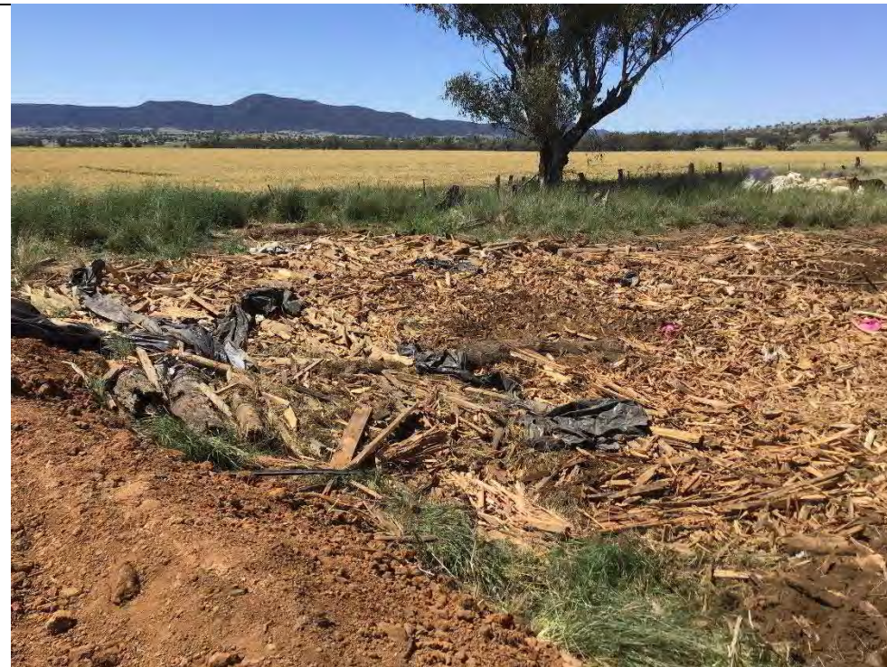
Photograph 22 – Timber stockpile spread and compacted into surface within the remediation area, facing north from adjacent TP202
