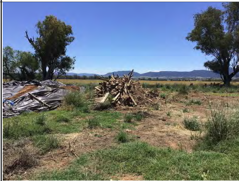
Photograph 19 – Timber Stockpile from demolition of sheep holding shed, facing north from TP201
