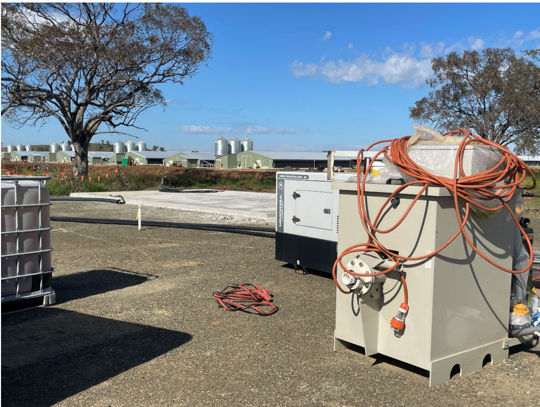
Photo 9: Water monitoring equipment on-site, to be installed.
