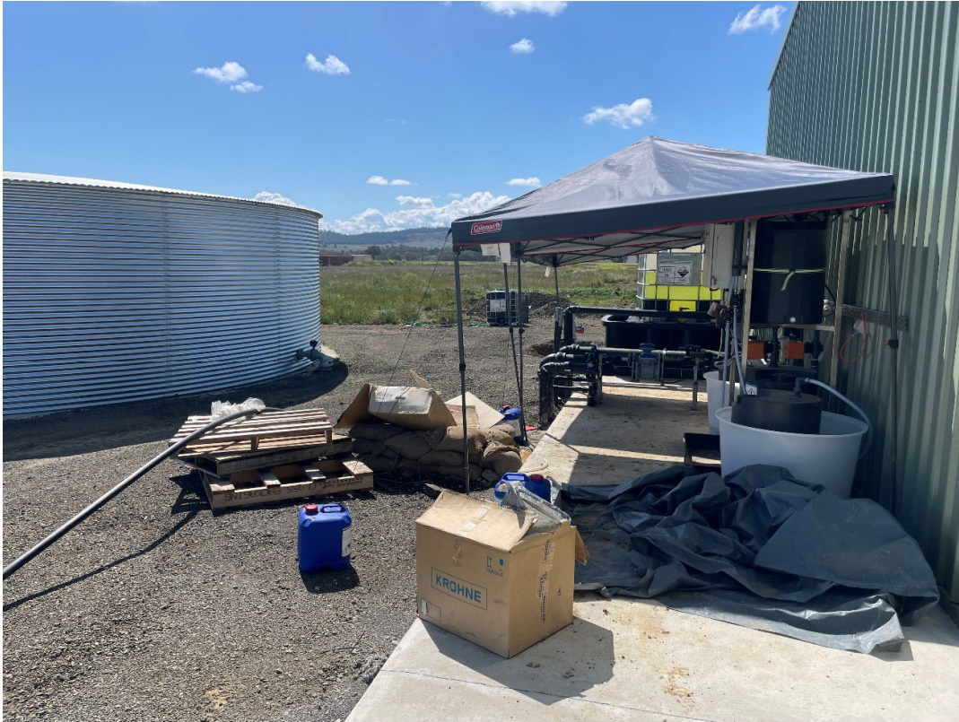
Photo 14: Water processing equipment in the process of being installed adjacent to the amenities/office shed.
