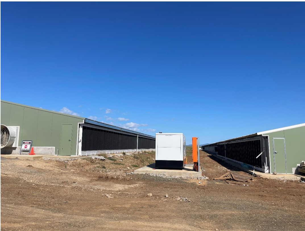
Photo 19: Generator between sheds.
