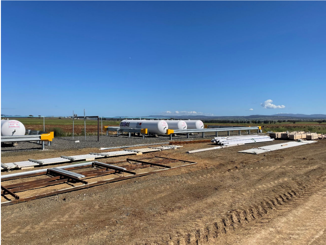
Photo 22: ELGAS tank area.
