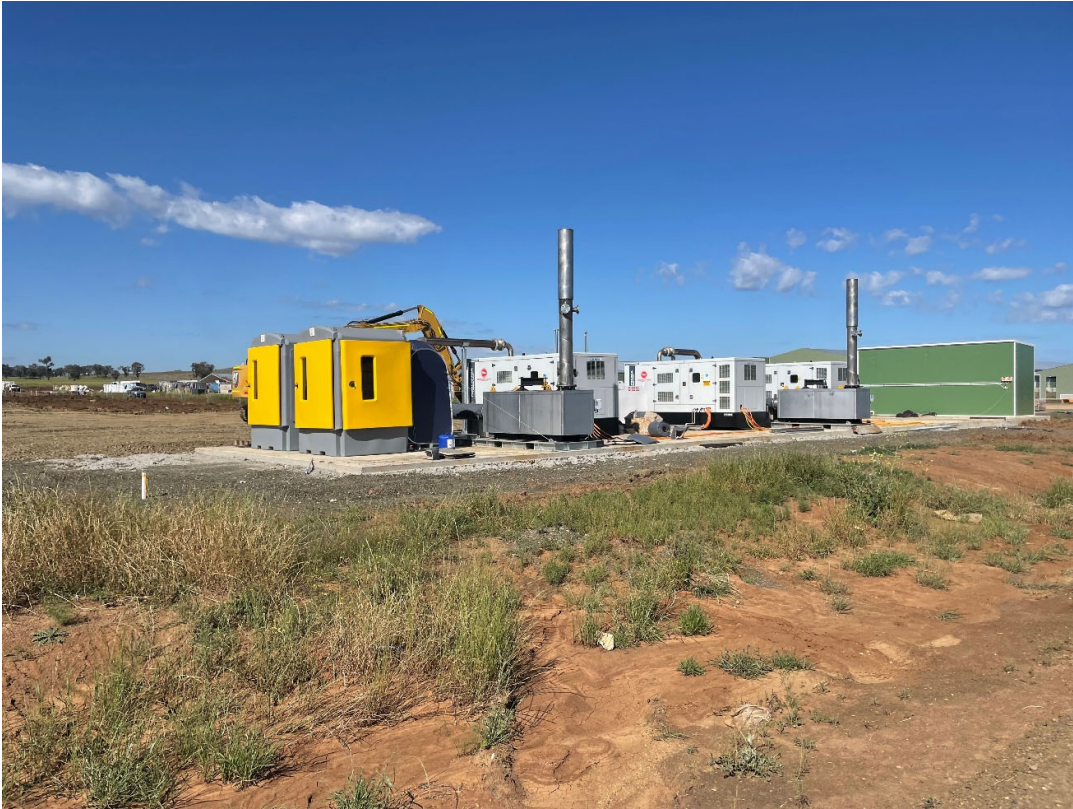
Photo 12: Enclosed diesel generators as power supply for Farm 2.
