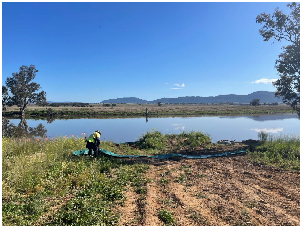
Photo 5: Repair of sediment fencing along Namoi River due to recent flooding in the Tamworth region.
