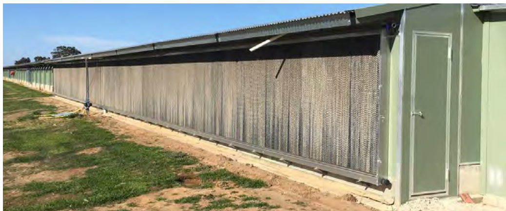
Photo 10 Side-wall cooling pad (ProTen's Narrandera Poultry Production Farm)
