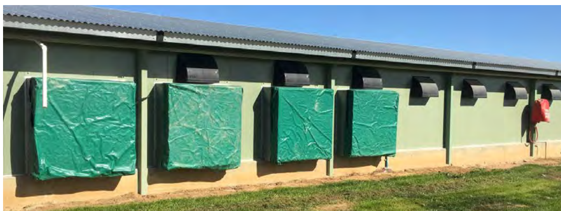
Photo 9 Side-wall fans (closed) and mini-vents (ProTen’s Narrandera Poultry Production Farm)
