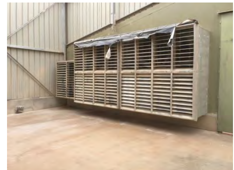
Photograph 2 Shed No.1 Exhaust Fan Release Point (at ground level)
