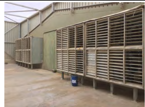
Photograph 1 Shed No.1 Exhaust Fan Release Point (at sampling ports/fan face)
