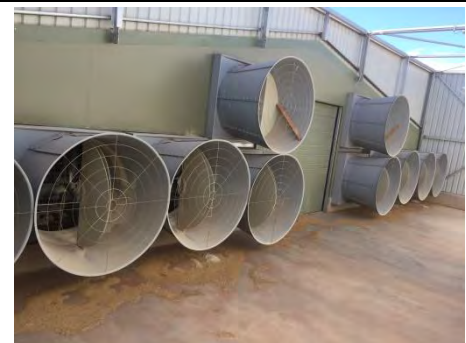
Photograph 1 Shed No.5 Exhaust Fan Release Point (at sampling ports/fan face)
