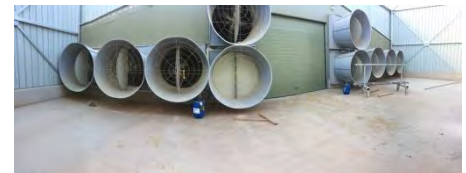
Photograph 2 Shed No.5 Exhaust Fan Release Point (at ground level)
