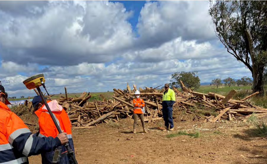
Figure 3 Timber from demolition of shed, to be used as capping material looking west. TPE facilitating the collection of GPS coordinates with the GPS Rover.
