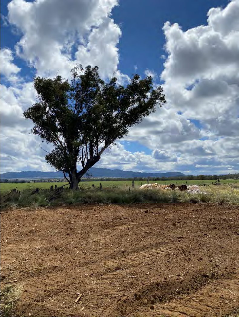
Figure 2 Soil on the footprint of the former shed after it had been demolished looking north east.
